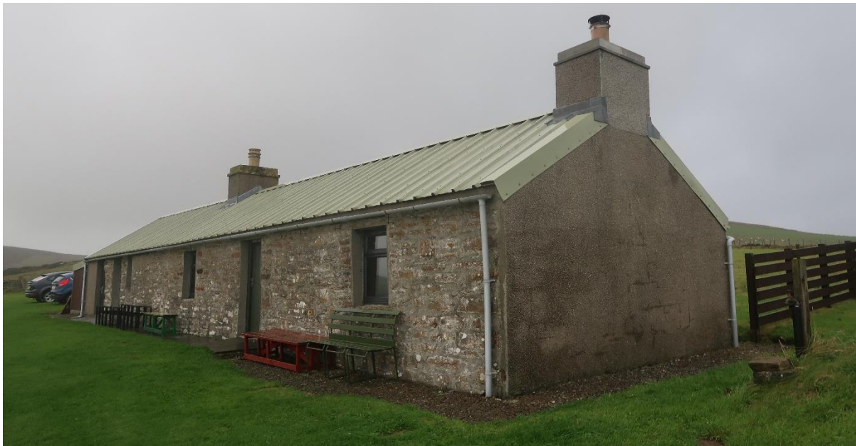
Fig 9, Gable elevation showing signs of dampness.
