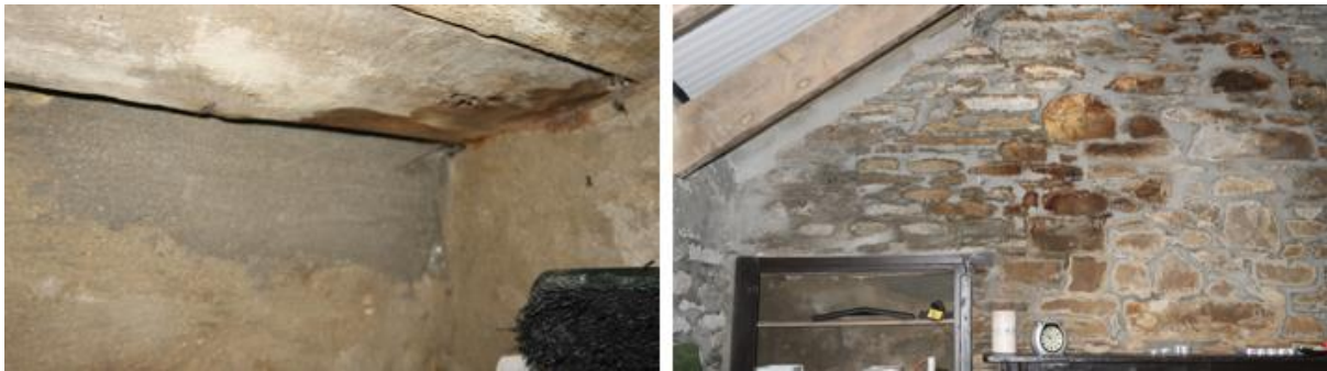
Fig 7: Photo of repair works carried out with non-porous materials & Fig 8 dampness of gable wall.
